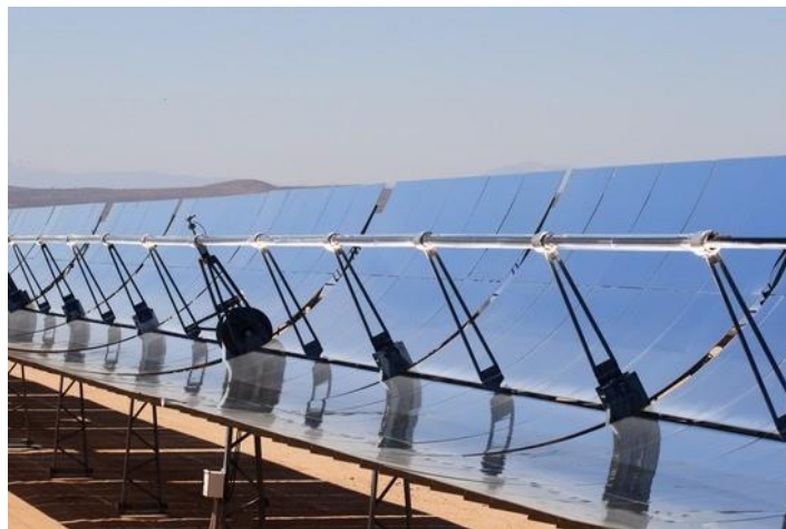
Figure 1. Parabolic trough solar concentrators (SEIA, No date provided)
